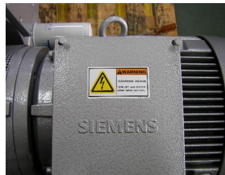
- Electrical Power inputting side -
